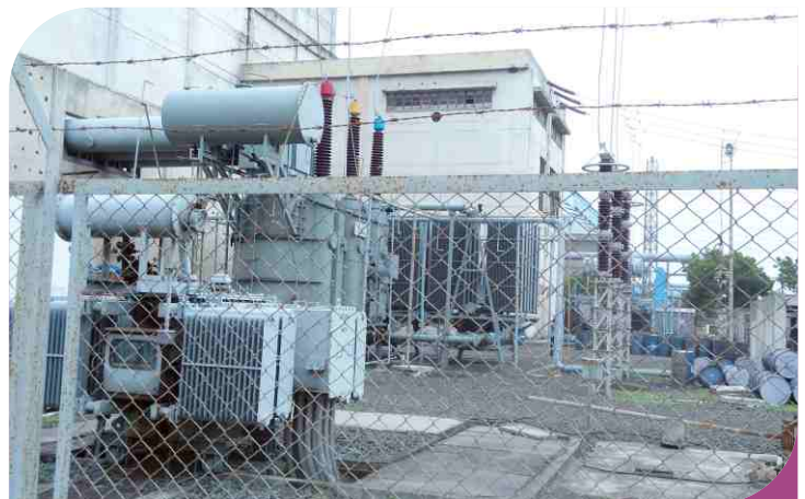
Getting acquainted with the step up transformer by the senior engineer of Sikka Power Plant
